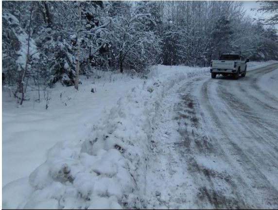
Ditches are needed above segment 135852 to transport water off the roadway.
