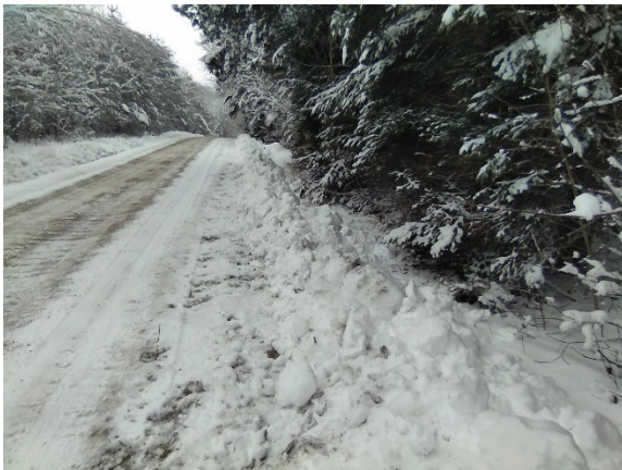
Ditches in segment 135852 are too shallow.
