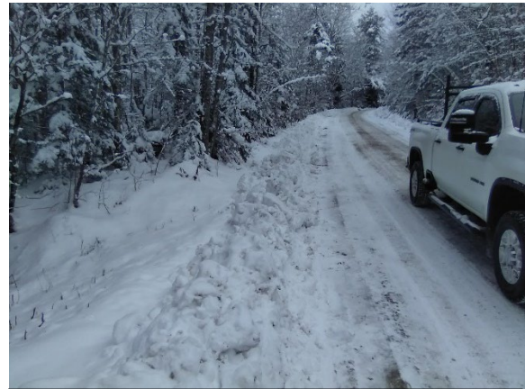
Ditches in segment 135851 are too shallow and not stone lined, resulting in erosion in the ditch.
