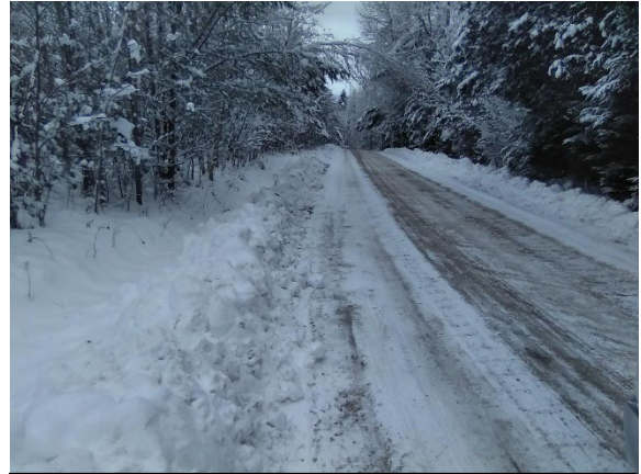
The crown in segment 135852 does not shed water evenly off the road surface, and ditches are not stabilized with check dams.
